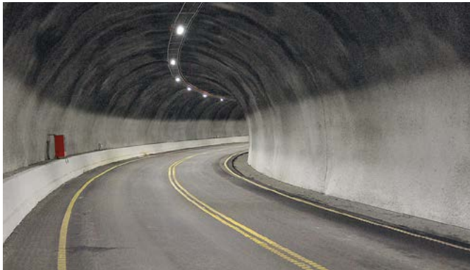
GTLED reduced energy consumption by 40% in Tinnsjø tunnels.
